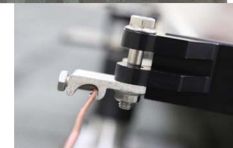
Install lay in ground lug with 5/16" stainless steel lag bolt, nut washer.
